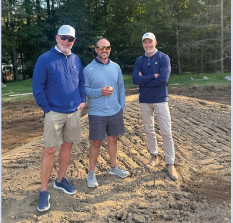
Bill Cygan reviews construction on Silver Spring's Hole #5 with greens chairman Todd Payne and golf course architect Brian Schneider.
